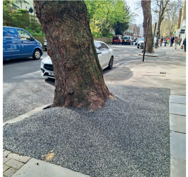
New resin bound tree pit around a mature plane tree on Hampstead High Street
